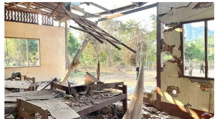
Image(8) – A high school building destroyed by the air attack
