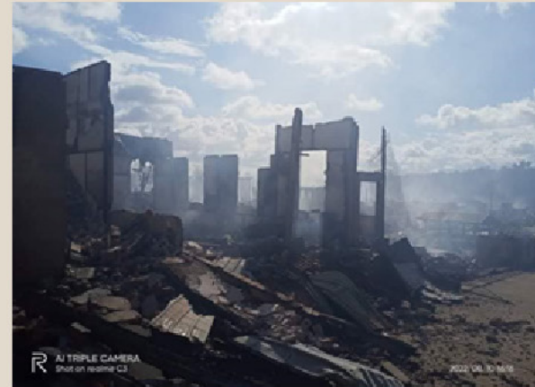
Photo - 2 A house burned down
