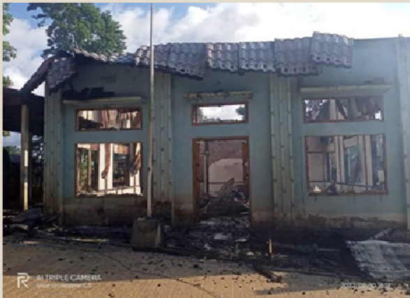
Photo - 3 A house burned down
